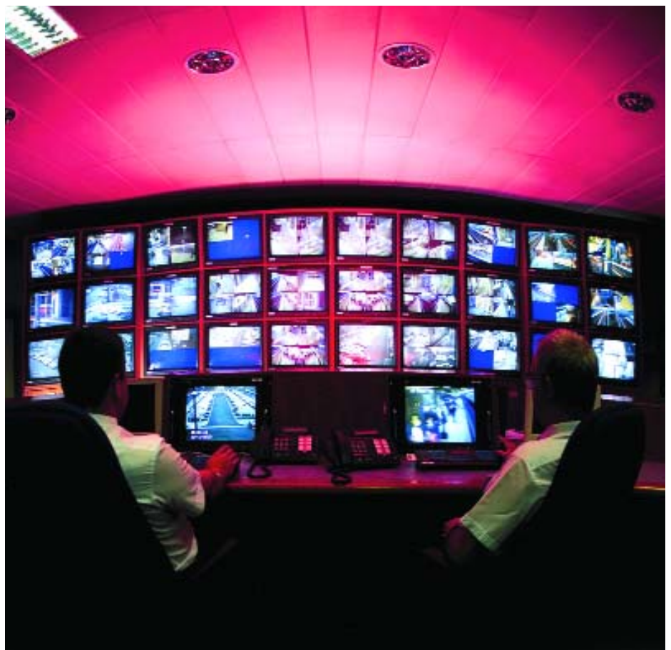
Centro's Network Safety and Security Control Room – CCTV images from hundreds of cameras are monitored here.
