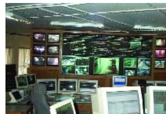
Manchester Metrolink Control Room.
