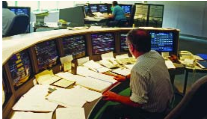
Control centres can look chaotic because staff need instant access to so much data.
