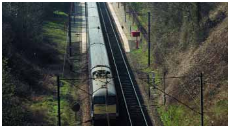
Electrification equipment is 30 years old on some parts of the East Coast.
